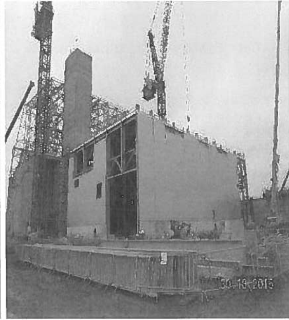
Turbine Hall (Copyright PML).
